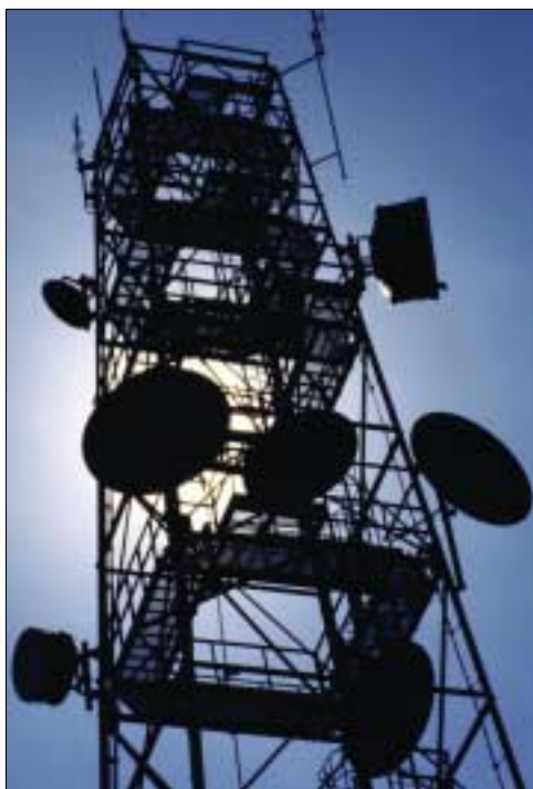
Network planning – the key to tomorrow's wireless infrastructure.
