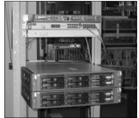
Figure 5. System hardware at the DeLeon central office.
